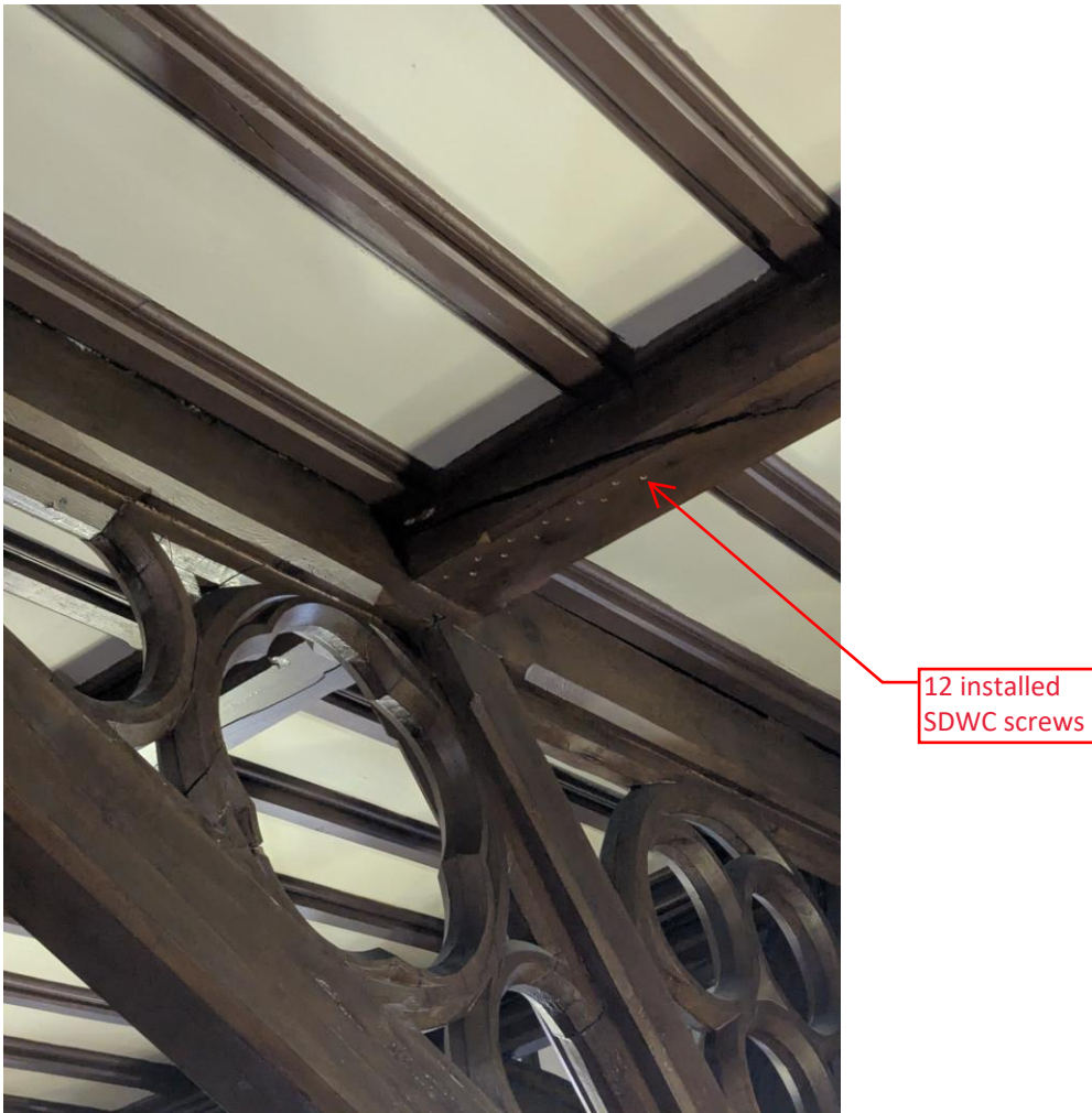
Picture 1: Shed roof purlin with fully threaded screws reinforcing cracked section
