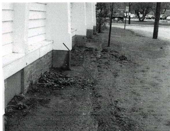
Figure 3 Moss and debris impede runoff
