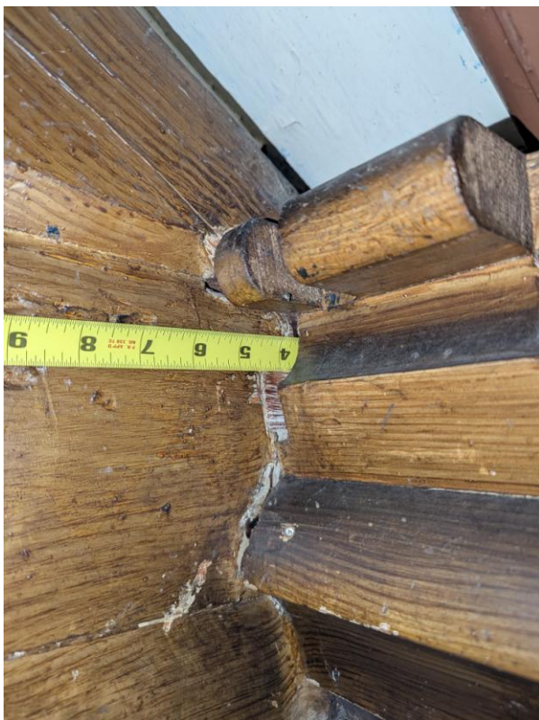
Picture 6: Bottom chord of shed roof truss extending beyond bolster block into eave wall
