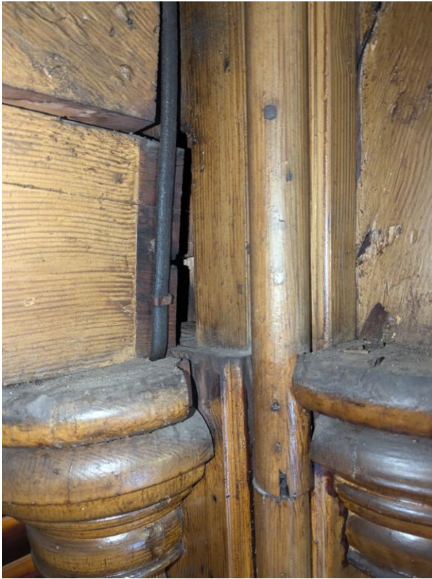
Picture 2: Bottom chord of shed roof truss has pulled away from center aisle post
