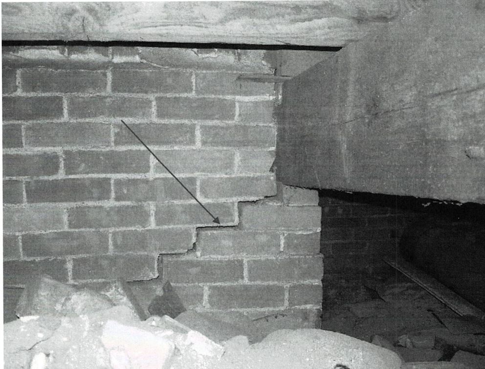
Figure 10 Bearing wall in failure.
