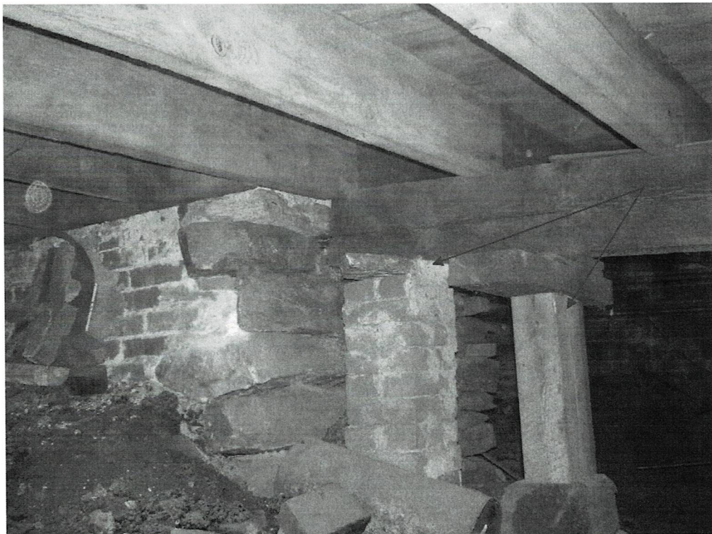
Figure 11 Bearing & Support lack fixity and lateral stability.
