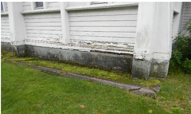
Deteriorated foundation at west façade
