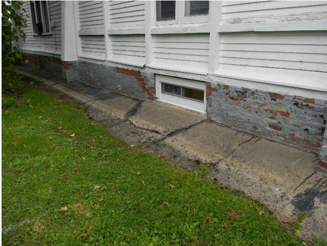
Deterioration at buttress bases, west façade
