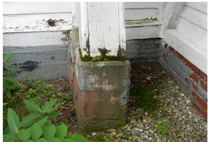
Deterioration at buttress bases, west facade
