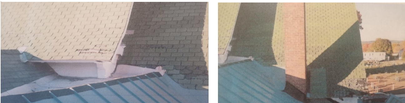
Photographs from 2016 inspection show complicated roof junctures and difficult drainage areas where Parish hall roof meets that of Sanctuary
