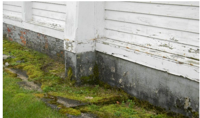
Deteriorated foundation at west façade
