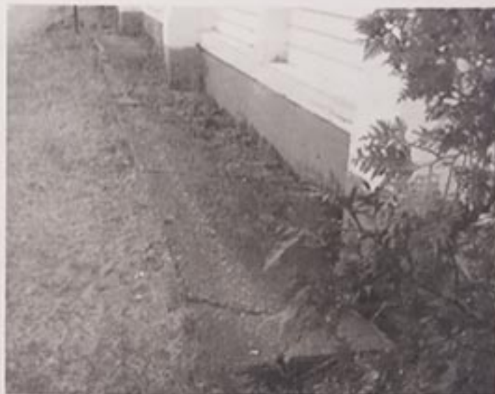
Figure 2 Northwest corner splash pad slopes toward building directing roof runoff to foundation.
