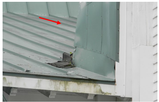
Dislocated shingles collecting at valley; Sheet metal improperly fastened and not sealed
