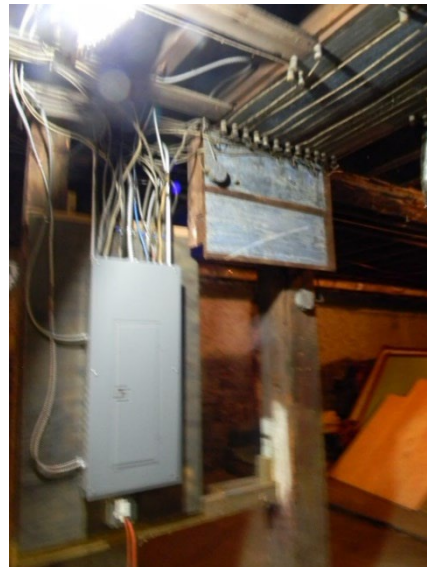
Mix of modern, 2-wire, and old knot-and-tube wiring
