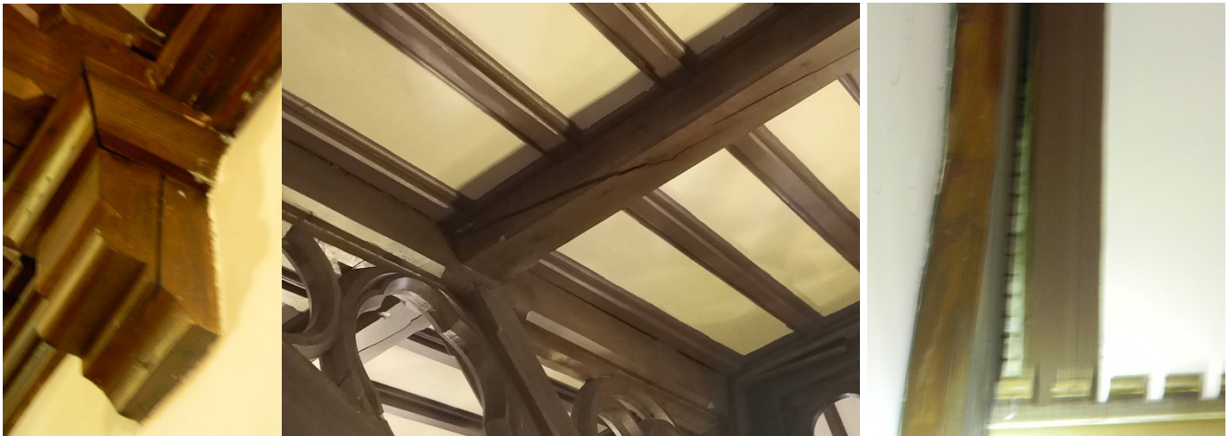
Cracking throughout the Sanctuary roof timber structural elements
