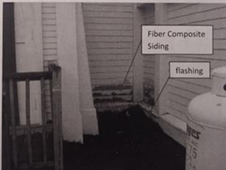
Figure 1: Flashing and siding maintenance have staved off deterioration in this wet area where paint won't hold but siding and sill are sound.
