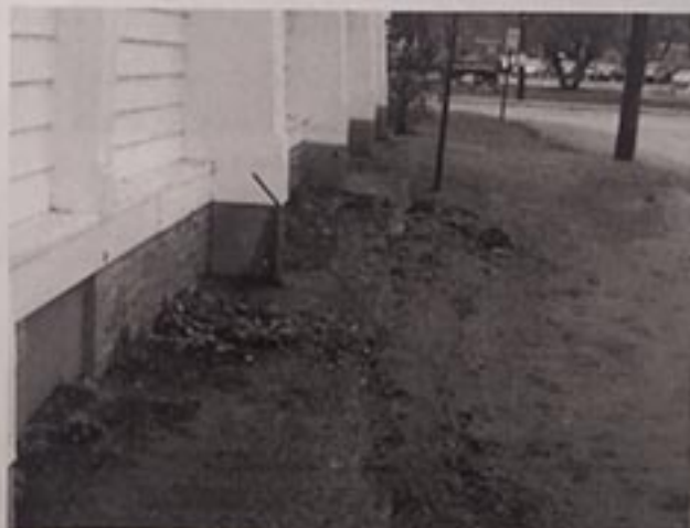
Figure 3 Moss and debris impede runoff
