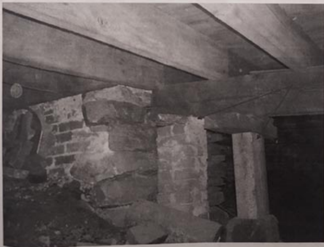
Figure 11 Bearing & Support lack fixity and lateral stability.
