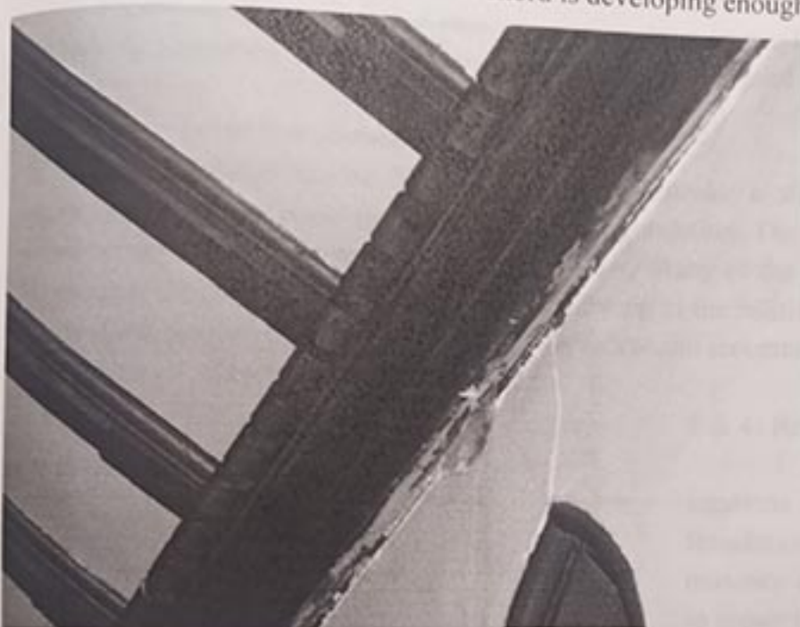
Figure 13 Loose Plaster at cornice, owing to the window size and shape, the plaster crack is no surprise.
