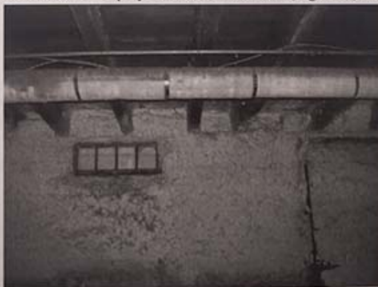
Figure 8 Insulation covers sill and wall but sill, joist and masonry resisted penetration wherever checked.
