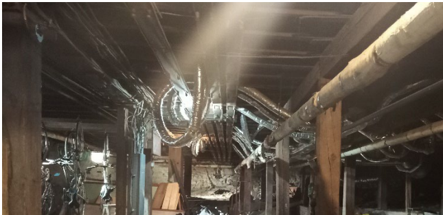
Flexible ducts supplying heat to the first few pews
