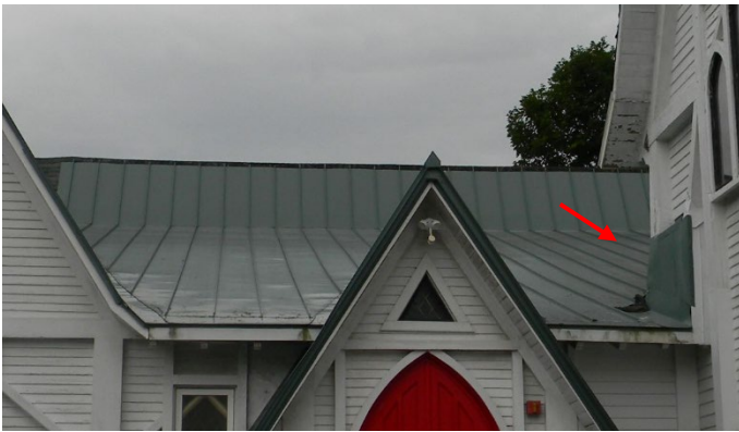
Isolated area of standing seam metal roofing at Parish; Water is directed at Nave wall.
