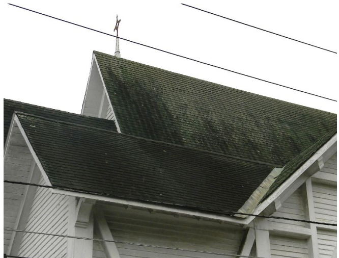
Black staining at north roof planes
