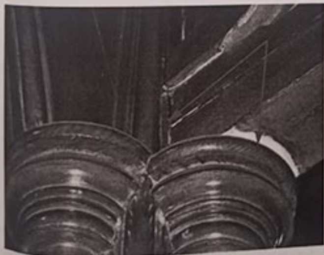
Figure 14 Lack of Stain suggests Bottom Chord has moved \frac{1}{2}'' to \frac{3}{4}'' . It is not clear how the chord connects to the Column.
