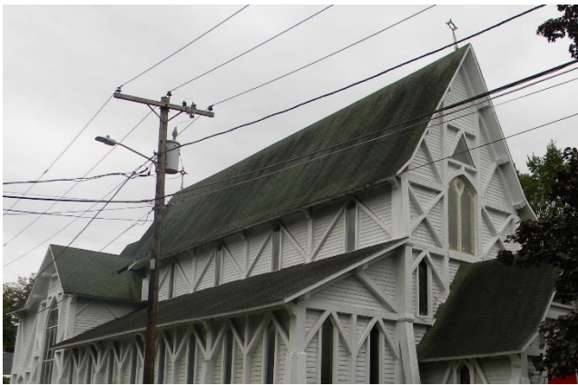
Black-staining, deterioration at north roof planes
