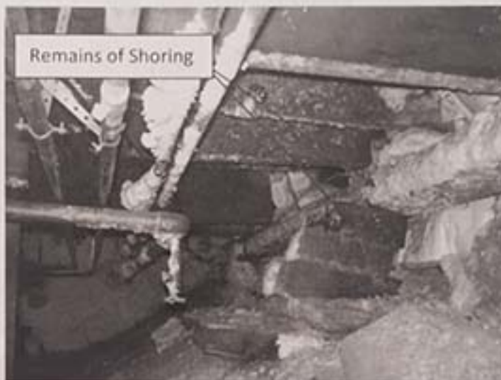
Figure 9 Plumbing, rubble, and insulation prevented closer observation of this north crawl space wall. Once shored these joist connections could not be observed
