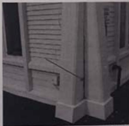
Figure 6 Separated cladding exposes timber column inside
