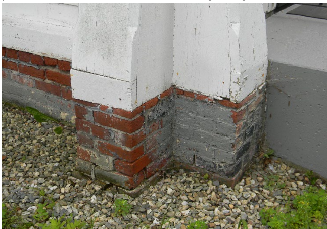
Deterioration at buttress bases, west facade
