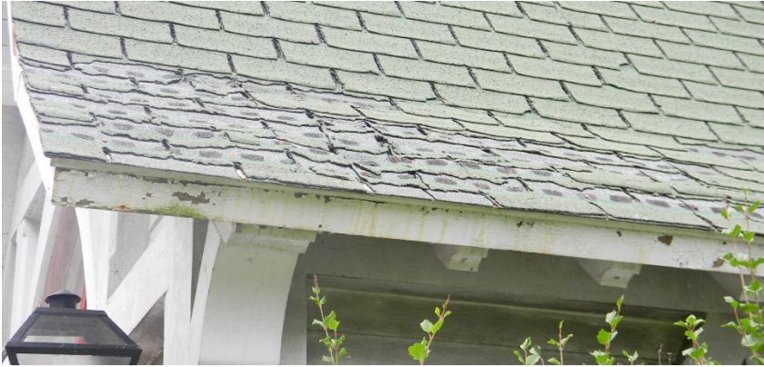
Deterioration, loss of granules at kicked eave
