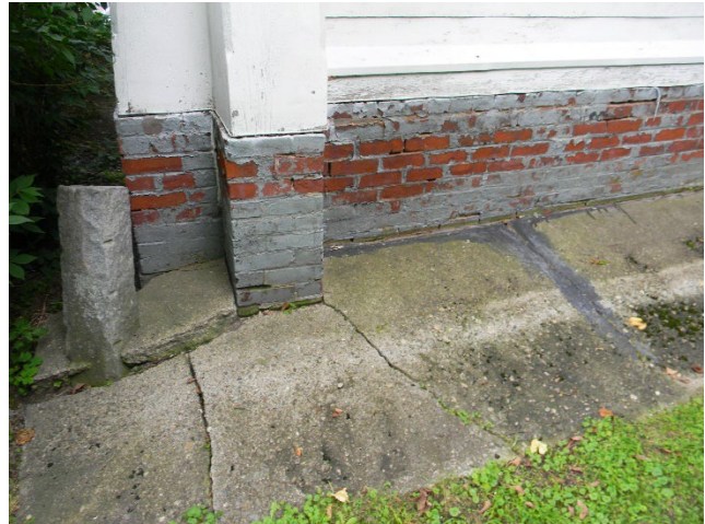
Deterioration at buttress bases, west façade
