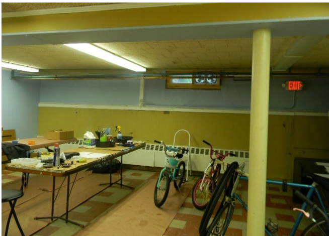
Staining and peeling paint was observed along the Chapel basement south wall.
