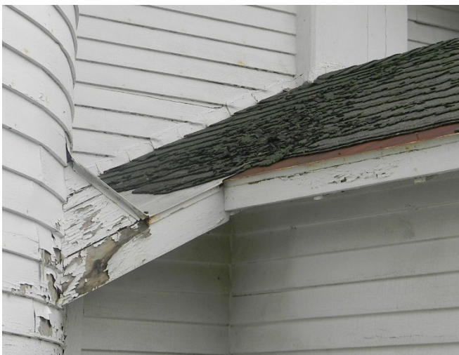
Deteriorated shingles at rear addition
